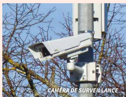
CAMERA DE SURVEILLANCE
